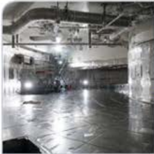
Emergency cooling water storage tank
