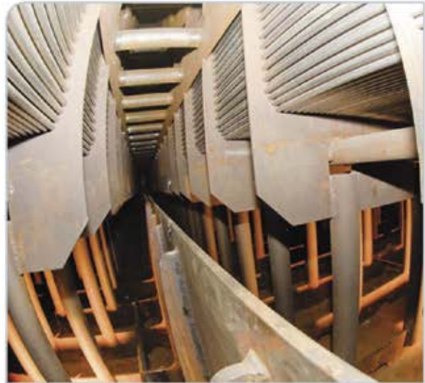
Condenser unit from the inside.
