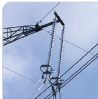
400 kV power line isolator chain.
