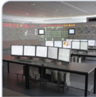
Simulator control room being tested in the manufacturer's facilities.
