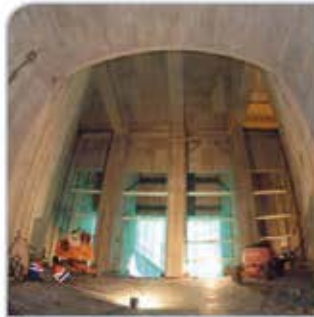
The cooling water intake tunnel has a cross-section of about 60 \text{ m}^2 .
