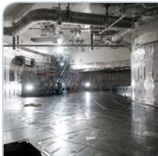
Emergency cooling water storage tank
