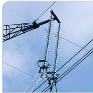
400 kV power line isolator chain.
