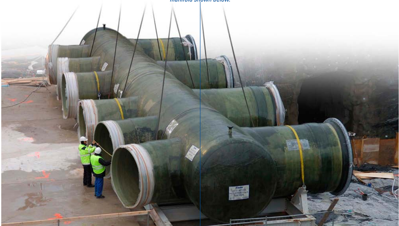
The cooling water pumped by the sea water pumps is conveyed into a sea water condenser through the manifold shown below.
