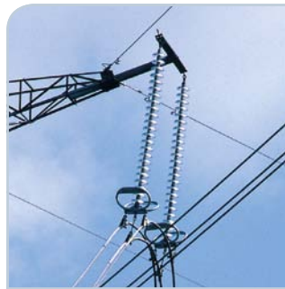
400 kV power line isolator chain.
