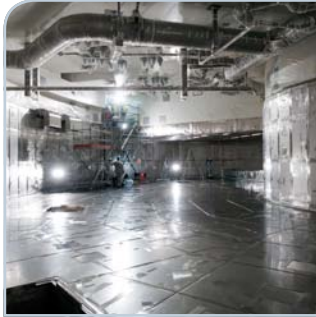
Emergency cooling water storage tank
