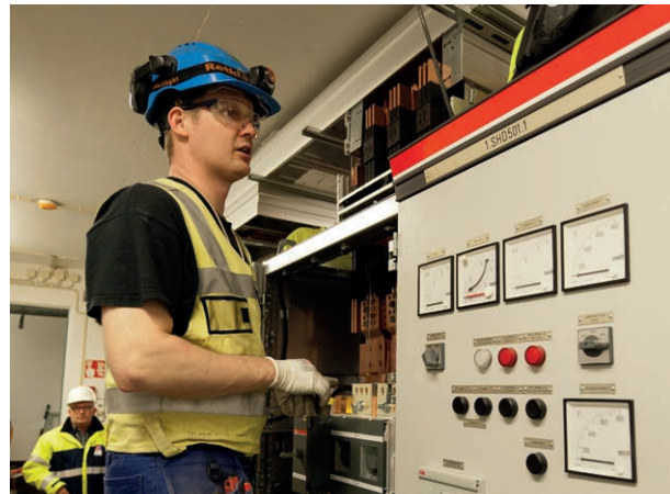
The main switchgear room of the diesel-backed system requires a space of about 150 square metres; this is a large system indeed.
