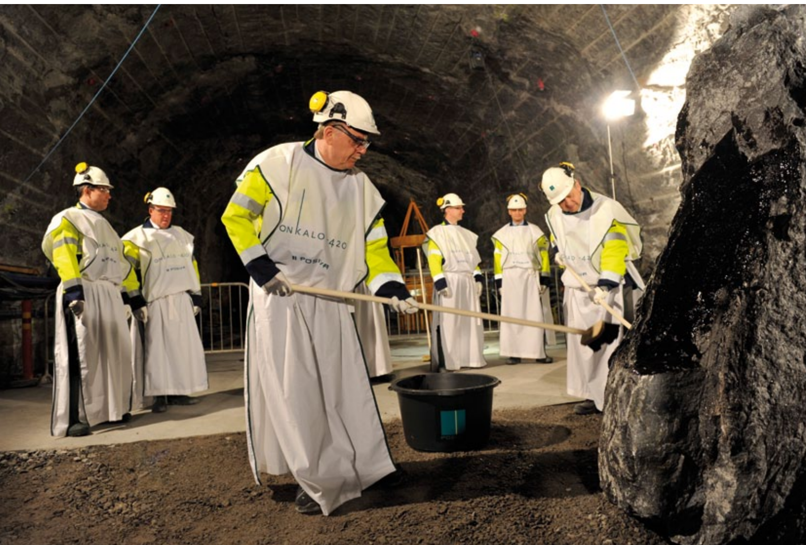
Topping-out ceremony at ONKALO on 17 June 2010. The tar brushes are wielded by Construction Director Pertti Huovinen (left) and Executive Vice President Timo Äikäs (right).
