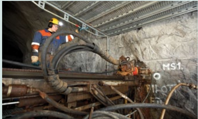
Boring of a test tunnel pilot hole at the disposal depth in ONKALO.
