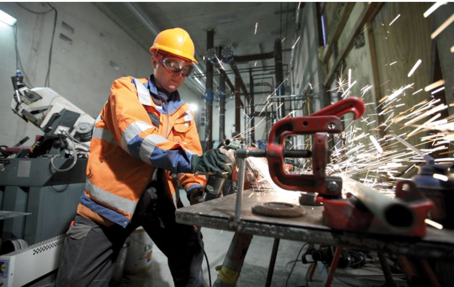
Work on the interior of ONKALO's ventilation building began towards the end of the year.
