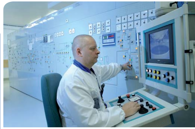
The ion-exchange resins used to purify the process water are solidified with bitumen and cast into steel drums. The bituminization process is controlled from the waste management building control room.
