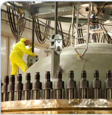
In the annual outage, new fuel is replaced in the reactor. Pictured: the reactor's cover.
