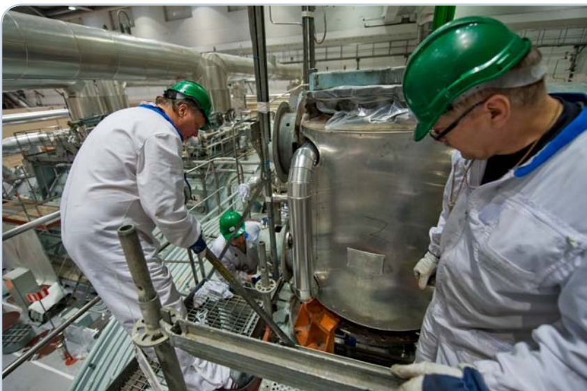
Renewal of the steam dryer has reduced the radiation levels of the turbine plant during annual outages.
