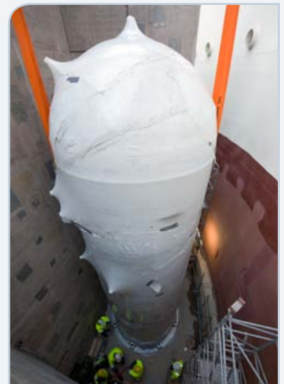
Lifting a Finnish-made pressure accumulator at the reactor plant. There are a total of four accumulators.
