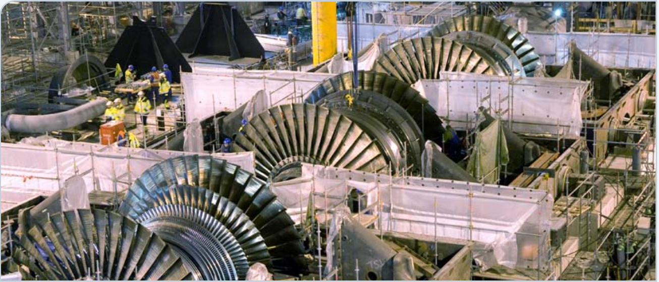
The turbines, the generator and the exciter have been installed at the OL3 turbine plant.
