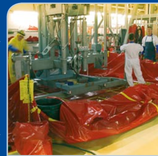
Employees at the unit wear protective clothing and accessories appropriate for the tasks. Work sites are always protected in accordance with the instructions provided by radiation monitoring.
